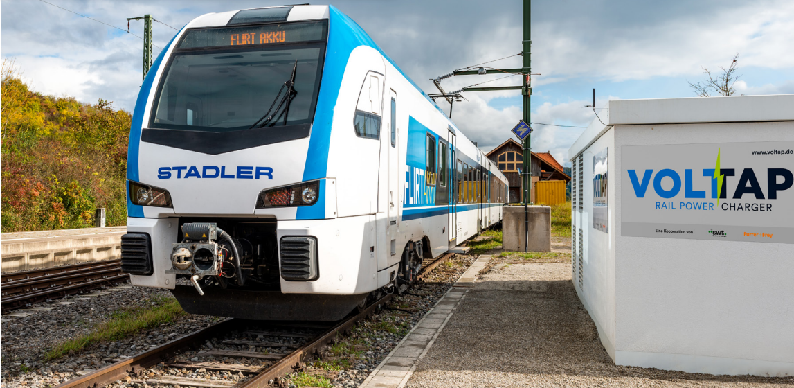
The VOLTAP rapid charging station consists of the transformer station (foreground) and an overhead line system (OLA) with charging masts and a charging rail. Photo: swt/Marquardt
